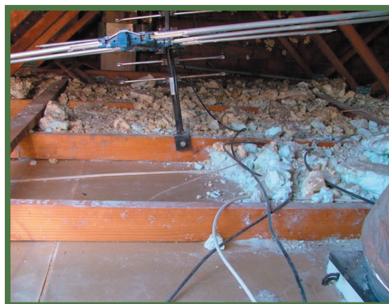
Degraded foam insulation
